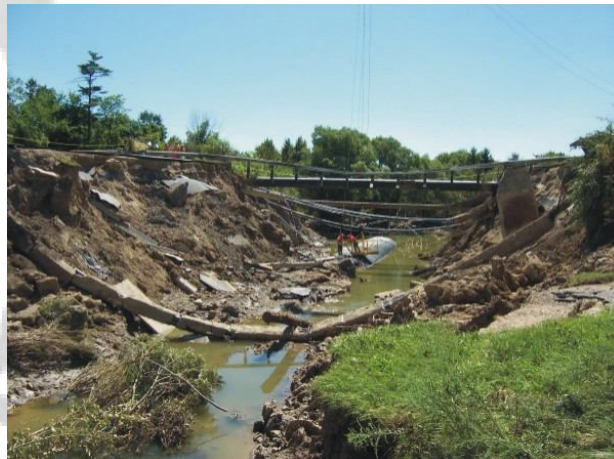
Black Creek Washout at Finch Ave, 2005.
